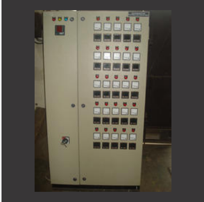
Electrical Heat Tracing Control Panels
