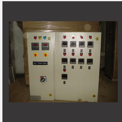
Heat Tracing Panel
