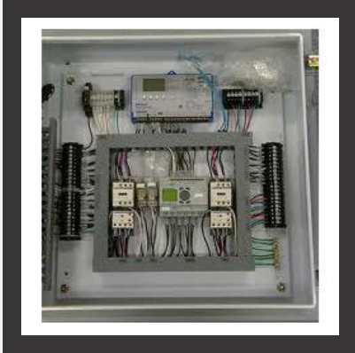
Electrical Control Panel
