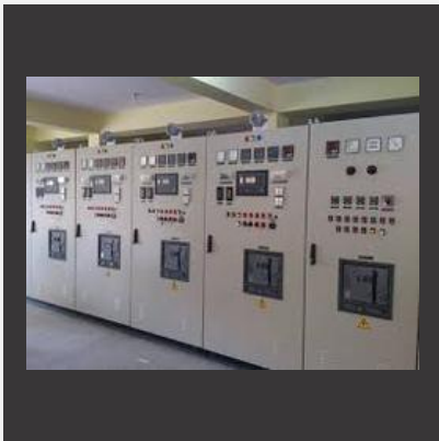
DG Synchronization & Distribution Panel
