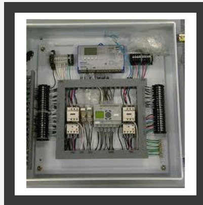
Electrical Control Panel
