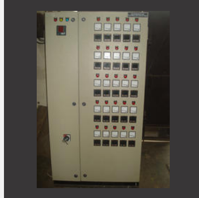
Electrical Heat Tracing Control Panels
