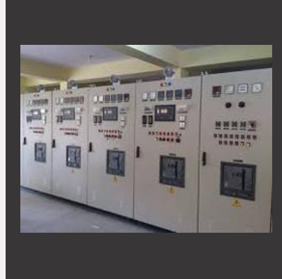
DG Synchronization & Distribution Panel
